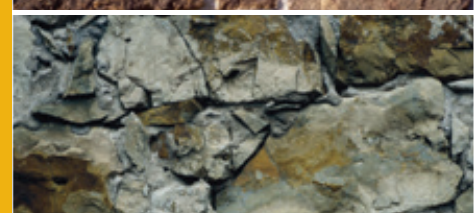
Top: Durable masonry with CALCIDUR®/HYDRADUR®; Bottom: Damaged masonry because of wrong binder
