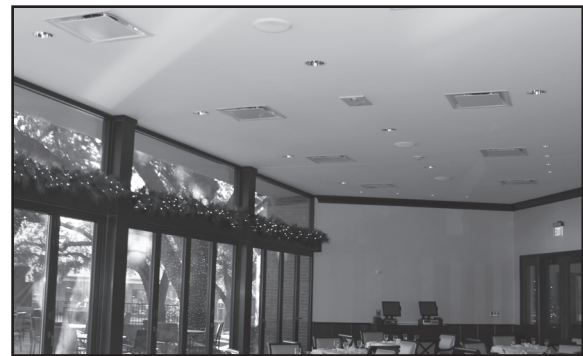
OMNI diffusers installed in the ceiling of a country club
