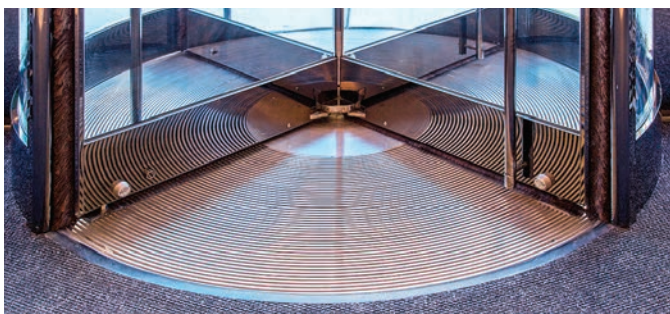
Welded Floor Grille
