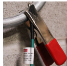
(3) Ground Pin Clamped On Metal Pipe.
