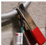
(3) Ground Pin Clamped On Metal Pipe.
