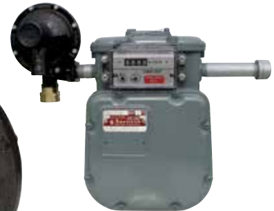
Attached to Vapor Meter
