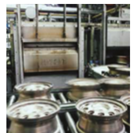
Aluminium age-hardening furnace with air/gas ratio controls for air deficiency cut-out
