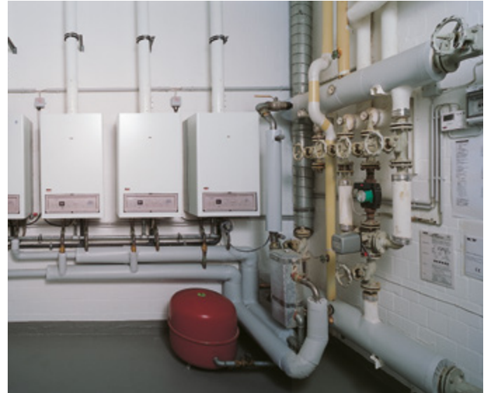
Heating boilers connected in cascade
