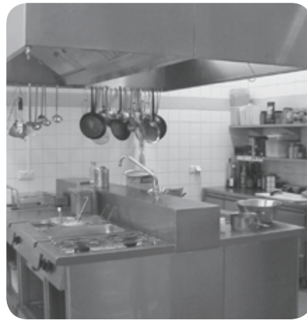
Filter monitoring in kitchens
