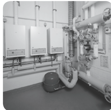
Heating boilers connected in cascade
