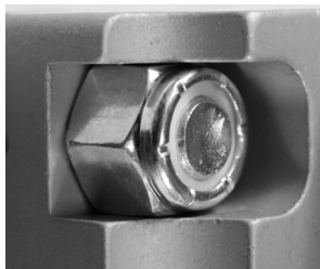
Fig 21 Bolt protrudes just beyond flush
