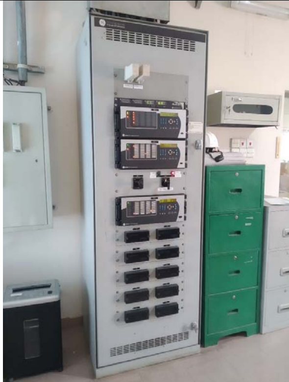
Protective Relay Panel
