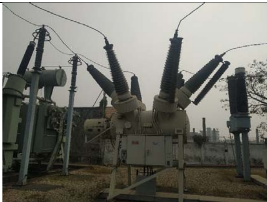
SF6 Circuit Breaker
