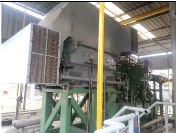
GBC (Gas Booster Compressor)
