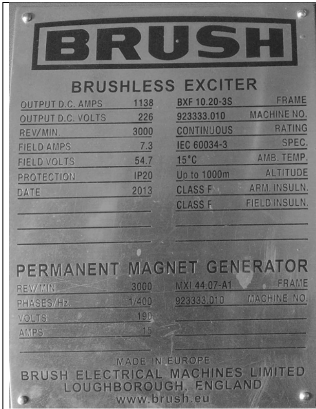
Generator Exciter Nameplate [At Actual]
