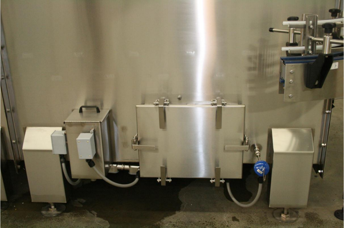
CLEAN OUT DOOR AND FLOAT BOX
