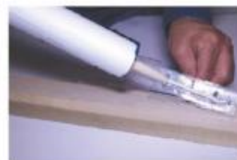
1) Put a moderate amount of sealant. 2) Align and press it on the surface. 3) Do the same process on the other rail.
