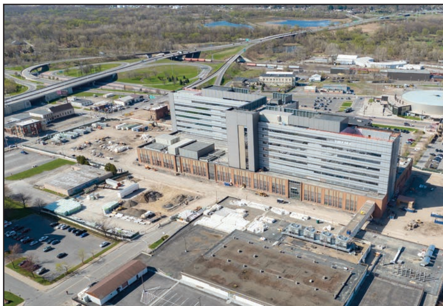
An April 30 shot of the new Wynn Hospital of the Mohawk Valley Health System that is under construction in downtown Utica.
