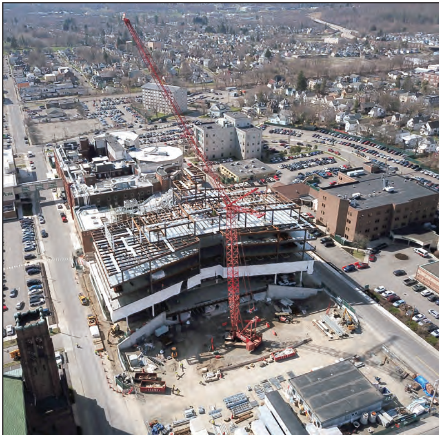
A recent construction photo of the UHS Wilson Medical Center’s six-story expansion project.
