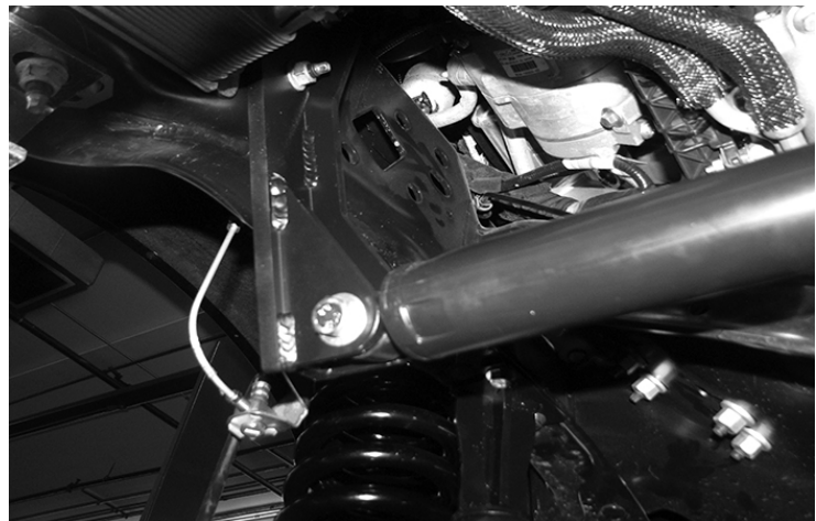
29. Remove the front sway bar from the frame mounts and save the hardware. (14-16) Install FT30630 (Driver) and FT30629 (Pass) using the the supplied 7/16 hardware.
