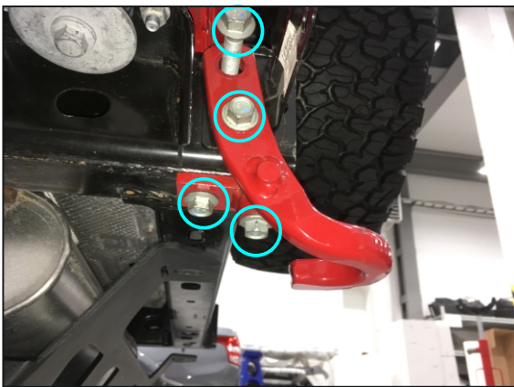
9. Unscrew OE tow hook's 4 fitting bolts on the left side of the vehicle. Set the tow hook aside as no further needed.
