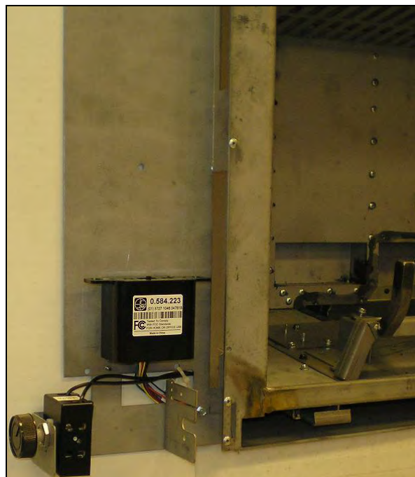
Components Out Remote Receiver Location.
