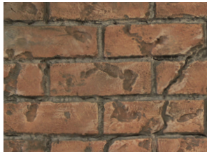
Fire Cracked Brick
