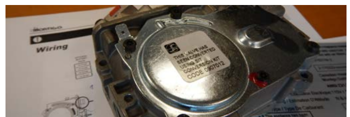
Figure 13.k Conversion label on valve
