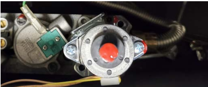
Figure 13.eee LP pressure regulator on a Full Load
