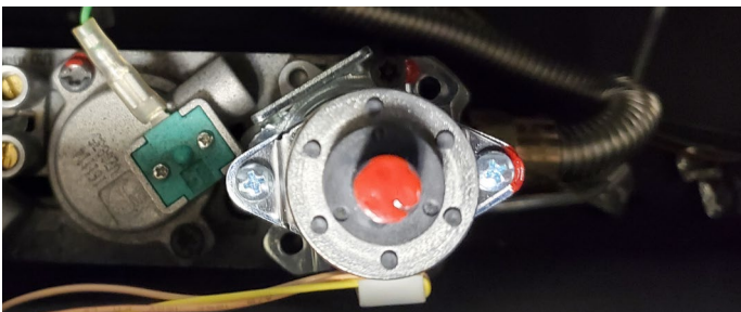
Figure 13.eee LP pressure regulator on a Full Load
