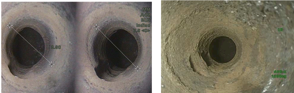
Figure 18. Damaged Radiation Shield Borescope
