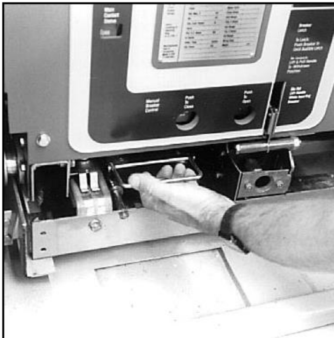
Figure 4-5 Pulling Secondary Disconnect Cage to Engage Secondaries in TEST Position (Old Version Shown). New Version will have BPI Pan With Automatic Secondaries.
