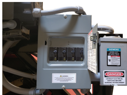
2 MAIN POWER PANEL & SWITCH
