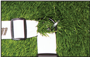
Step 3: Pull tight, slightly stretching the material, and anchor the first corner ring to the ground. Repeat this process until the entire GRID perimeter is outlined.
