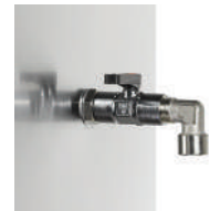
BLOW DOWN VALVE
