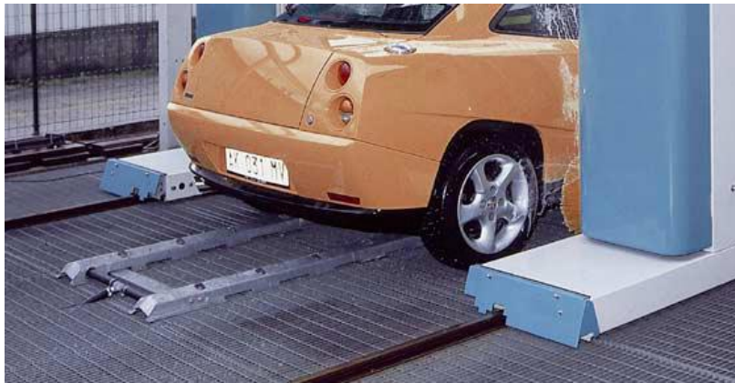
9882- Under chassis wash
