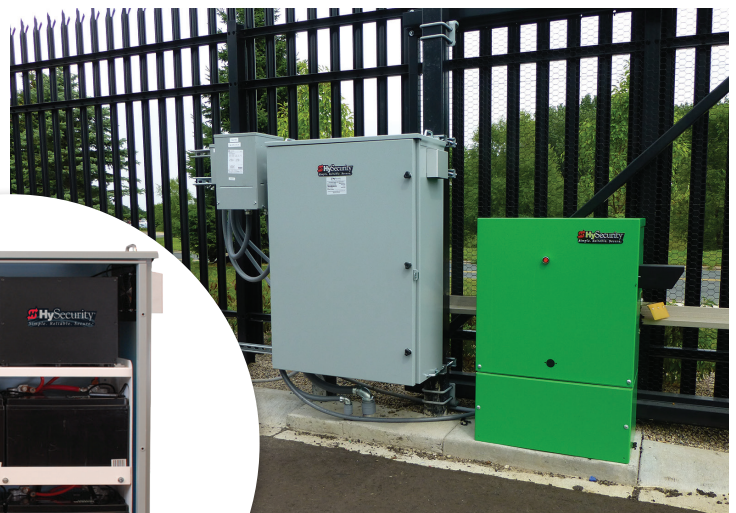
SlideDriver 50VF2/3 at Data Center
