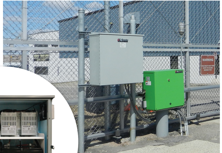
SlideDriver 40 UPS at aviation facility
