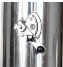
Damper lever in Closed Position
