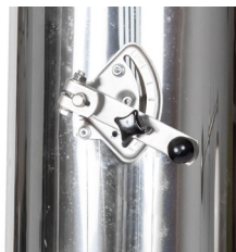
Damper Lever in 10% open Position
