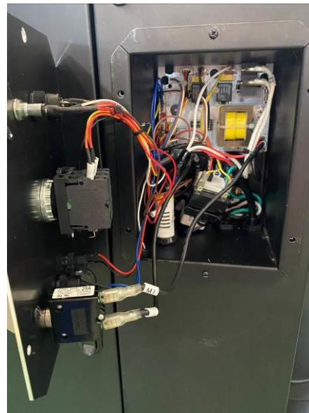
Figure 8: Control Panel/Box Wiring
