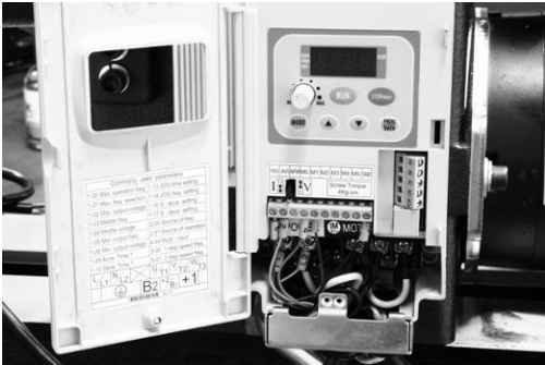
VFD with cover open
