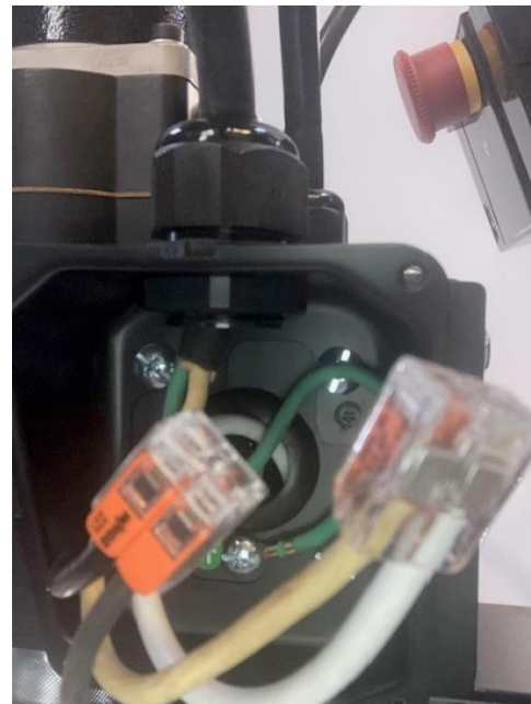
Fig. B. Installed Wiring
