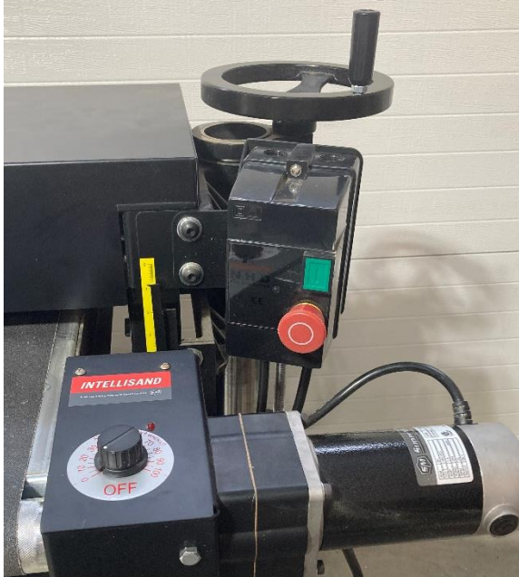
Fig. 31. Conveyor control box (Intellisand) and on/off switch.
