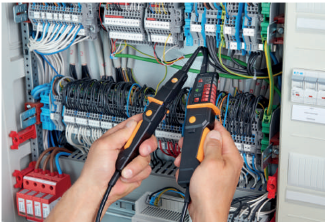
Measuring voltage in a switching cabinet.
