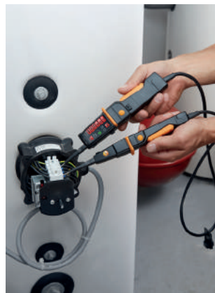
Measuring voltage on a boiler.
