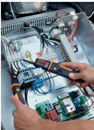
Measuring voltage on a compressor.
