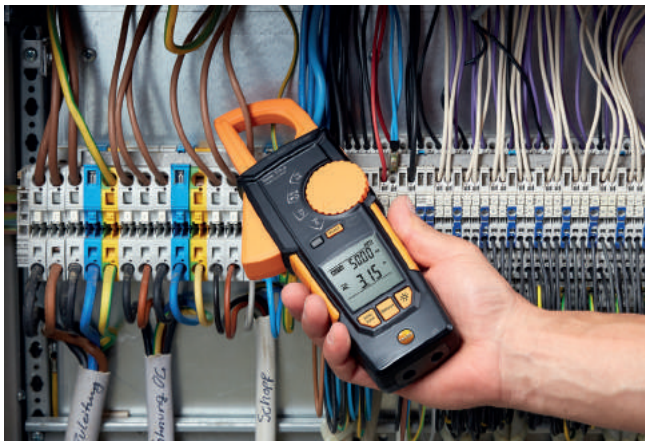
Measuring current in a switching cabinet.
