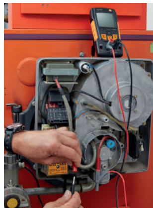
Ionization current measurement set-up
