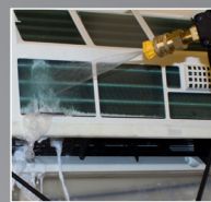
Clean coils from the front
