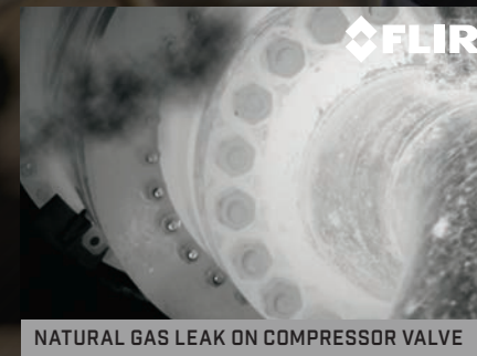
NATURAL GAS LEAK ON COMPRESSOR VALVE
