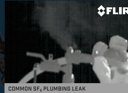
COMMON SF 6 PLUMBING LEAK
