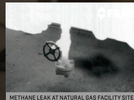
METHANE LEAK AT NATURAL GAS FACILITY SITE
