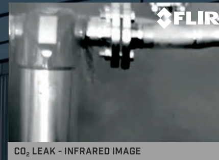
CO 2 LEAK - INFRARED IMAGE
