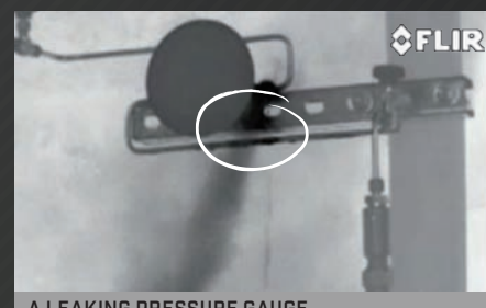
A LEAKING PRESSURE GAUGE
