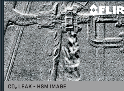
CO 2 LEAK - HSM IMAGE
