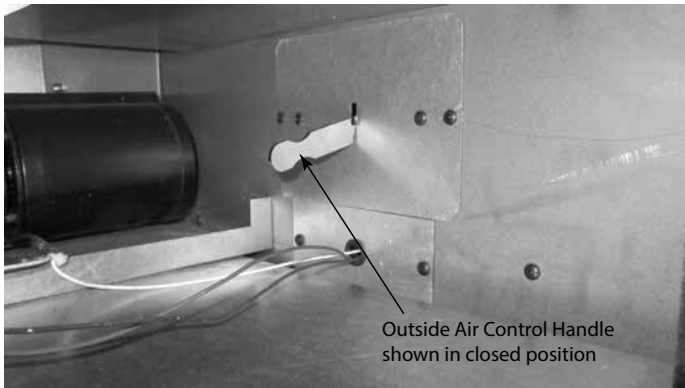
Figure 3.20 Outside Air Handle Shown on Right Side
