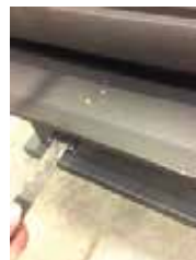
Air control for heat output
