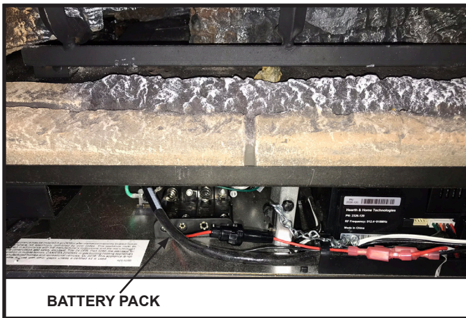
Figure 6.3 Battery Pack Installed
