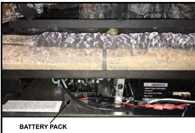
Figure 3.8 Battery Pack Installed
