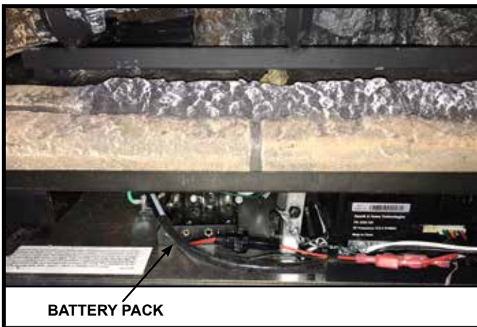
Figure 6.3 Battery Pack Installed
