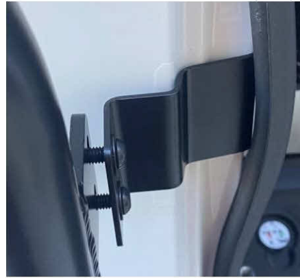
Figure 16: Example of gap between bracket and rack
