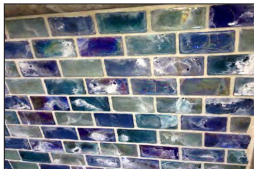
Example of glass failure due to no expansion joints.
