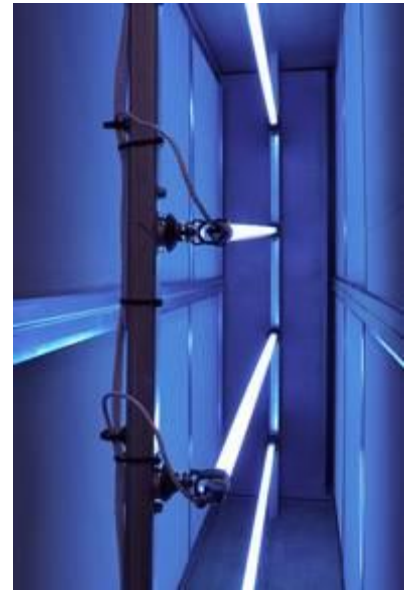
V-PAC Installation Barona Resort Casino San Diego's Leading Casino Resort
