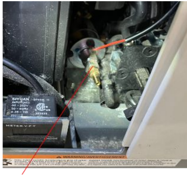
Fuel pump with outlet hose removed
