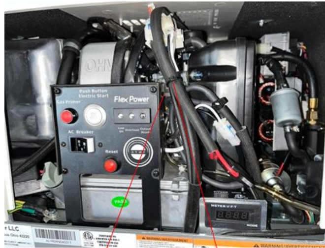
Carburetor (behind this bundle)
