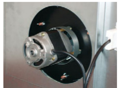
The fan on the back of the boiler.
