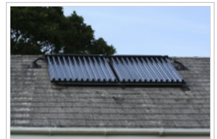
Vacuum Tube Panels on a roof
