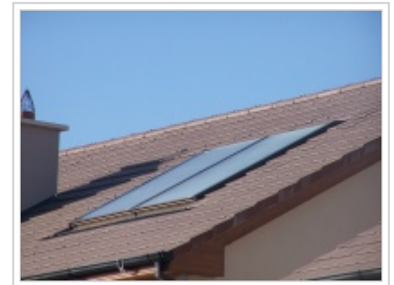
Flat Panels on a roof
