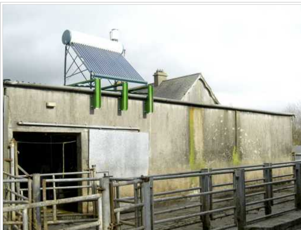
Solar Water Heating System installed on roof of Dairy.
