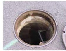
Missing manhole covers and floor sections
