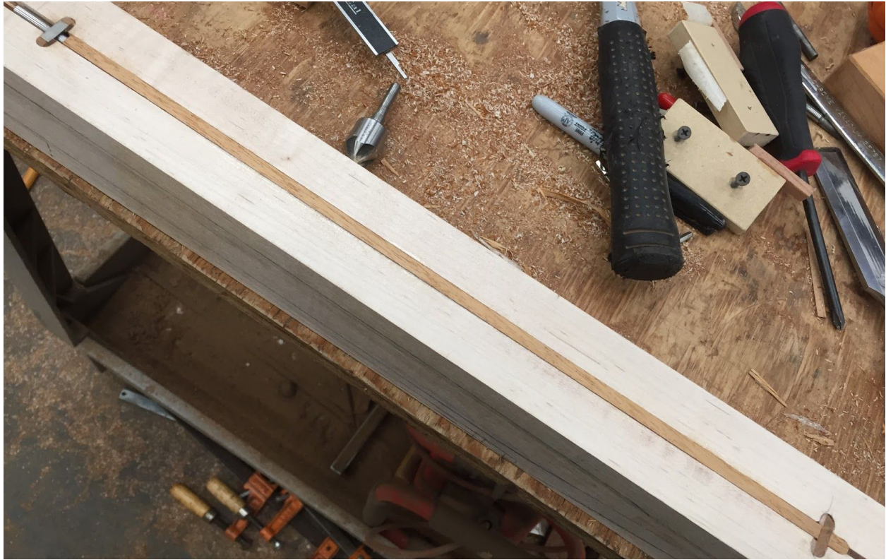
29. The installation is complete.
